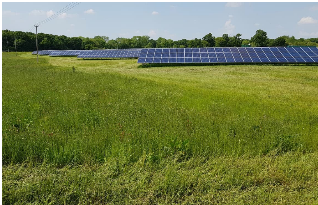
Plate 1: Landscaped Solar PV Facility
