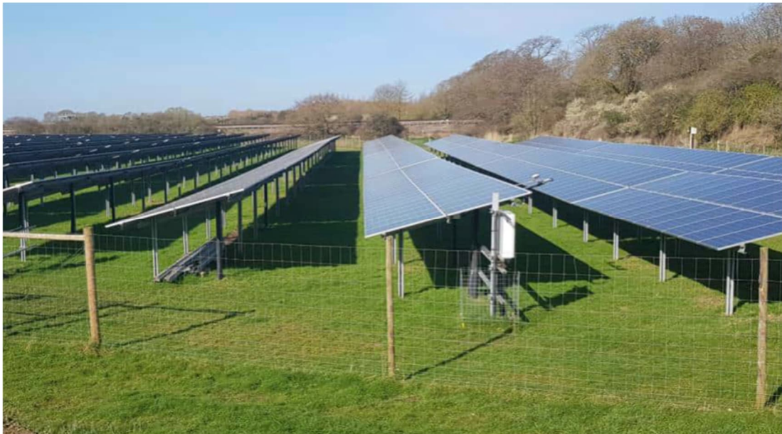
Plate 2: Example South Facing Solar PV Panels
